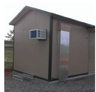
Electric Sub Station
