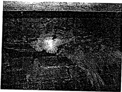
Mold growing around vents and along foundations.
